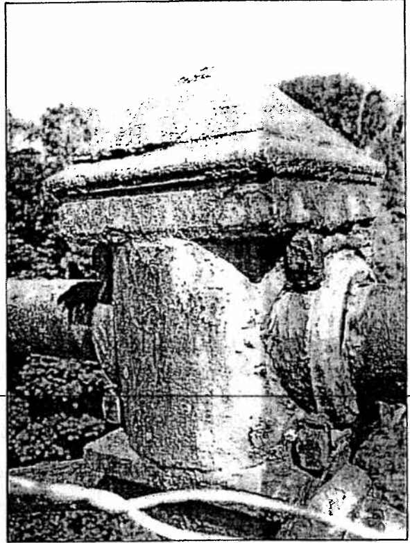
Inappropriate Repairs and Eroded Paint
