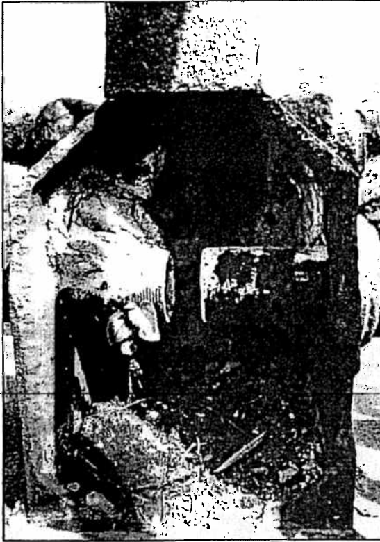
Spalling Cast Iron at Post Base
