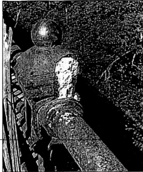
Spalling at Post Cap Due to Grouting of Post and Ice Jacking
