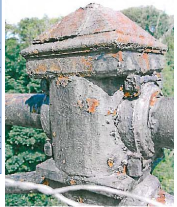
Inappropriate Repairs & Eroded Paint
