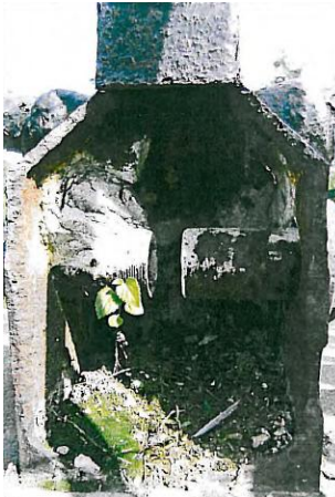
Spalling Cast Iron at Post Base
